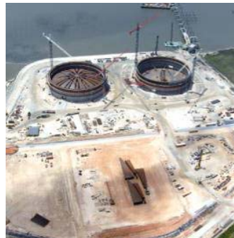
Gulf LNG EPC project on US Gulf coast, in joint venture with IHI. Receiving terminal for LNG shipped from around the world, helping supply energy to the Southern states of the US.
