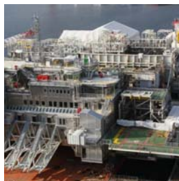
The Gjøa topside currently under construction at the Stord yard in Norway.
